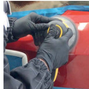
Sand damaged area using P320. Clean with Silicone Remover and apply plastic adhesion promoter.
